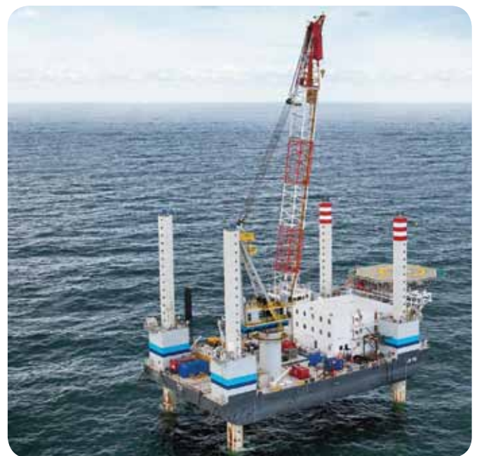
A marine exclusion zone will apply around the jack up barge at all times during construction.
