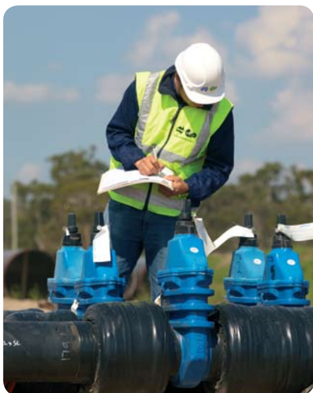
Crews will inspect the pipeline to ensure it is performing as required.
