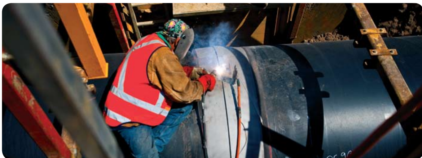
Minor construction work will connect sections of pipeline that have been successfully hydrotested.
